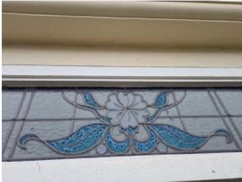
Photo 3 - Faded floral section and deterioration to other sections over door
