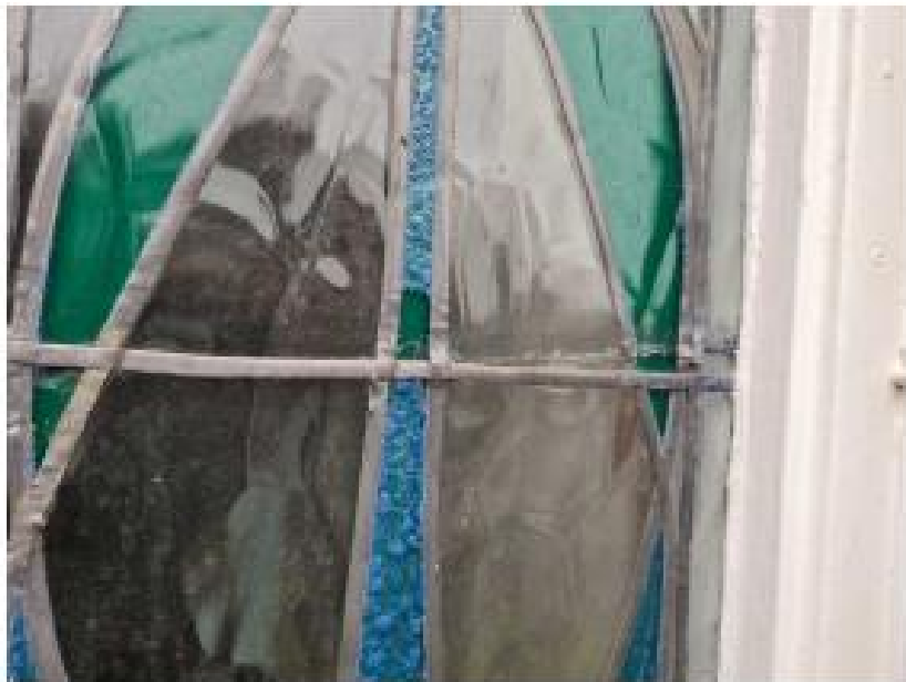
Photo 4 - Break in glass pane
