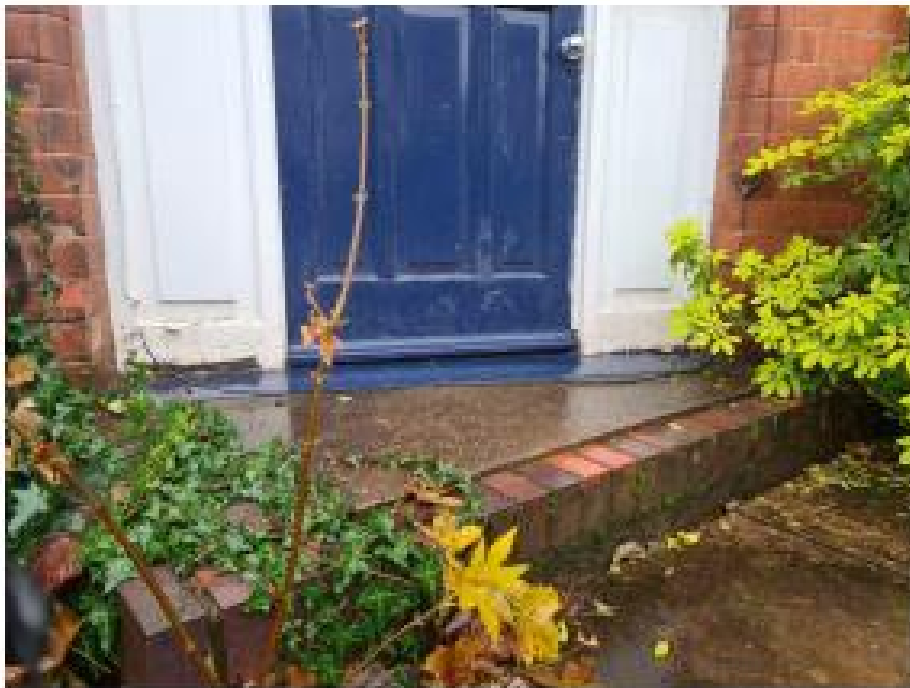
Photo 1 - Gap underneath door allowing water ingress into the building
