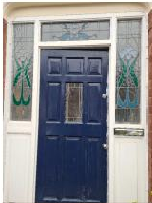
Photo 2 - General view of doorset. Note fading and unevenness in colouring to glass panels either side of door
