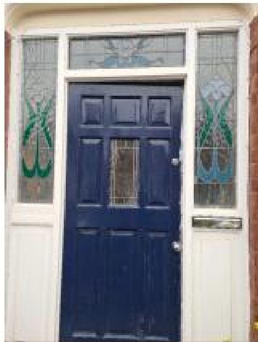
Photo 2 - General view of doorset. Note fading and unevenness in colouring to glass panels either side of door
