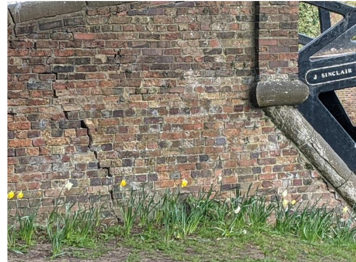
Figure 28: Cracks to Brickwork
