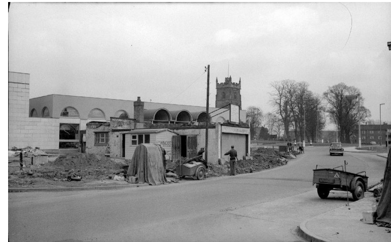
Figure 9: Abbey service station in Church Street, during demolition. This was in front of the newly constructed Public Library 18
