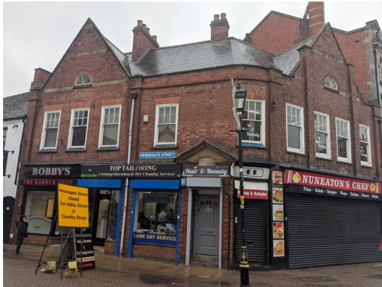
Figure 72: Signage not in sympathy with the host building
