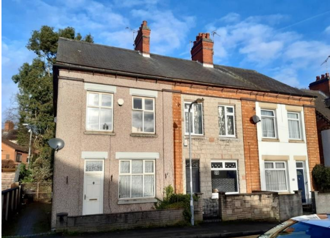
Figure 66: Satellite Dishes, Exposed Wires, Cladding
