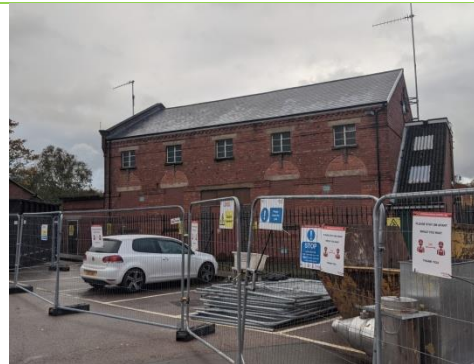
Sub Station rear of Town Hall
