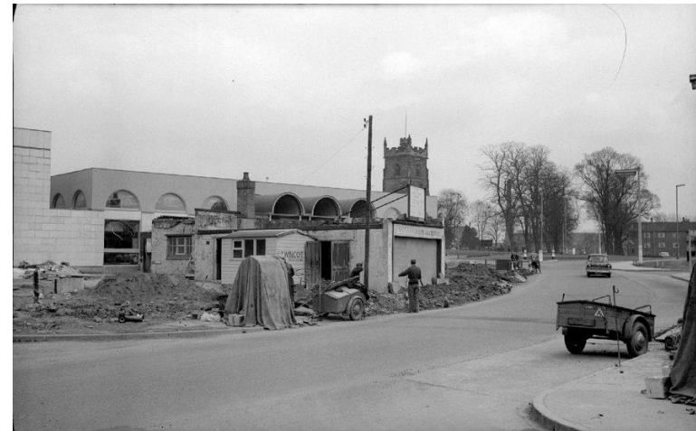
Figure 12: Abbey service station in Church Street, during demolition. This was in front of the newly constructed Public Library 18
