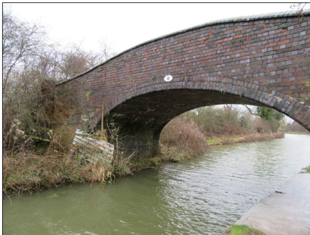
Plate 11: Detail of Bridge 18 of Coventry Canal, located in between strategic sites HSG3 and EMP1.
